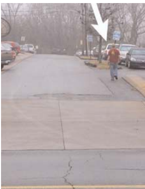
Exhibit 5-44. Lack of a sidewalk forces the pedestrian into the driveway.
