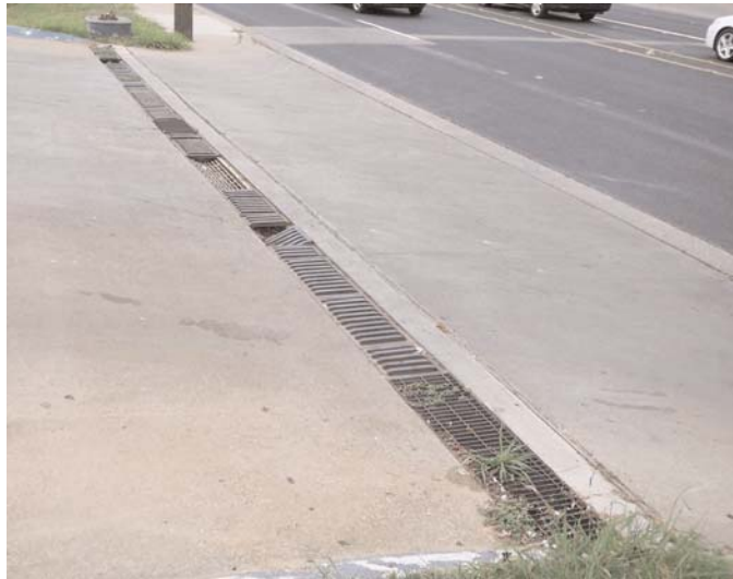
Exhibit 5-80. Damaged grates in driveway need repair.
