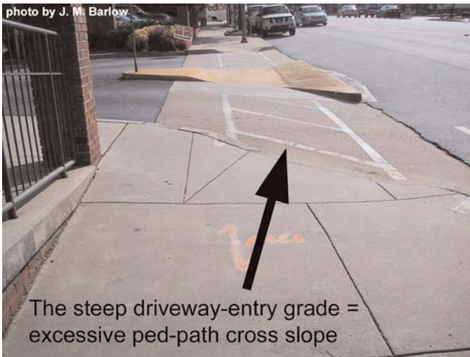
Exhibit 5-62. Example of driveway grade creating unacceptable sidewalk cross slope.
