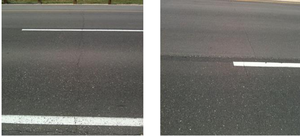
Figure 44. Longitudinal joint performance for the IA 13 project
