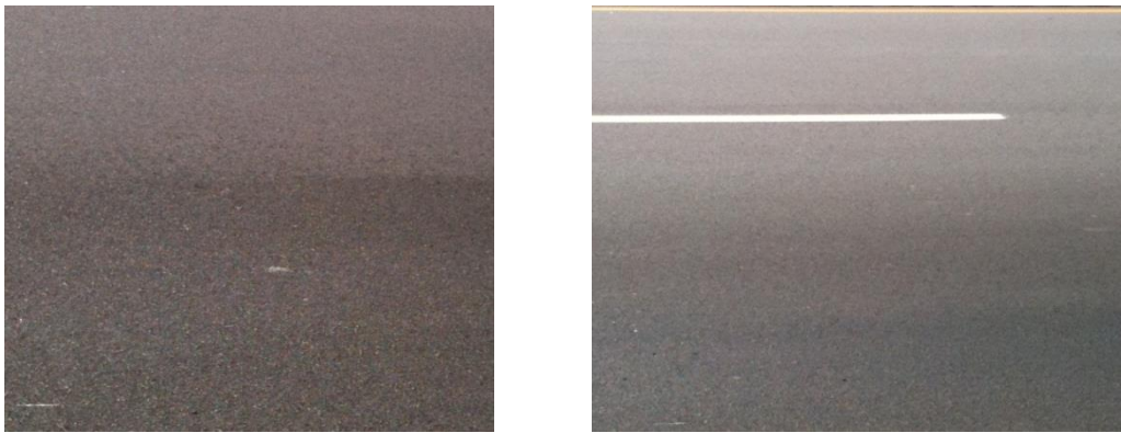
Figure 45. Longitudinal joint performance for the I-35 project
