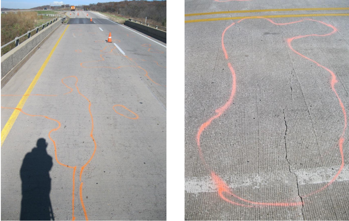
Figure 3-3 Photographic Documentation of Delamination
