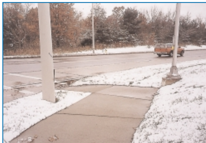
It is all too common to see sidewalks that end abruptly.
