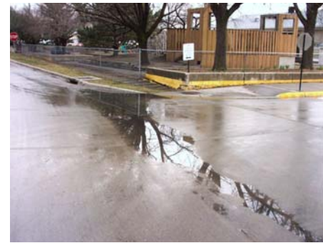
Flow line lower than intake
