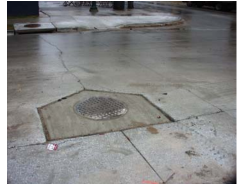
Crack resulting from poor jointing around utility access boxout
