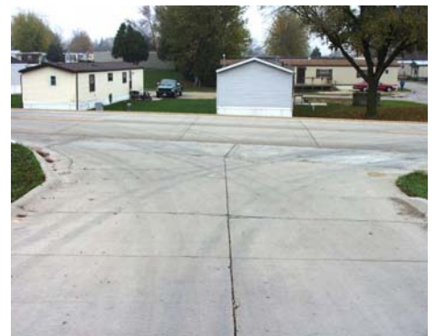
Driveway joints don't match the highway joints
