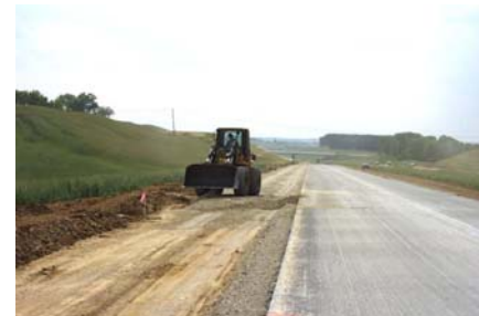
Outlet covered with granular material
