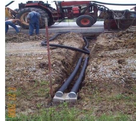
Subdrain outlet on patio blocks
