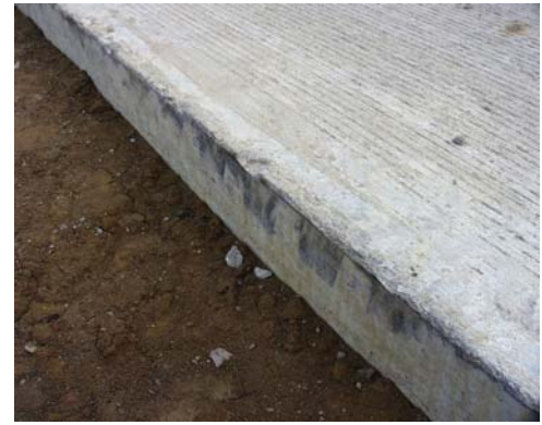
Chipped slab edge from finishing equipment
