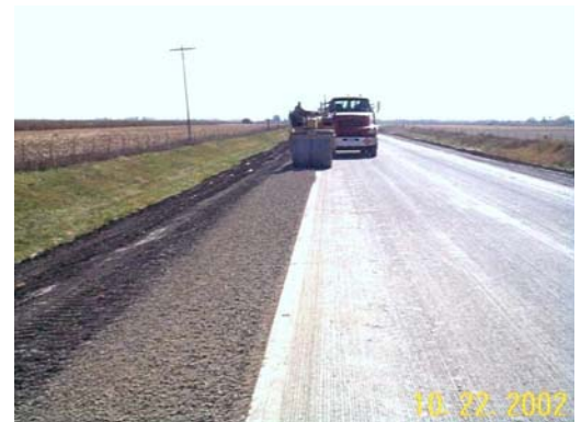
Roller partially on the slab likely causing chipping of the edge
