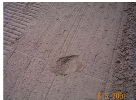
Fine material on the surface due to segregation
