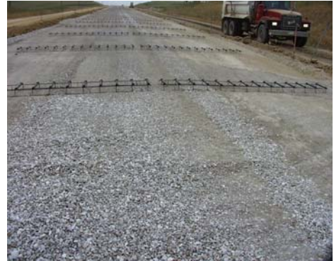
Variability in material due to segregation during trimming
