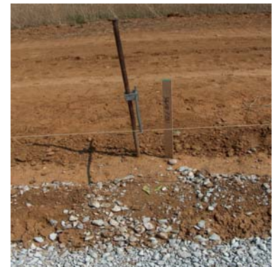
String line can be a tripping hazard
