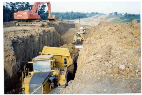
Unsafe conditions need to be reported
