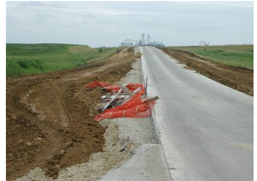
Safety closure removed from closed roadway
