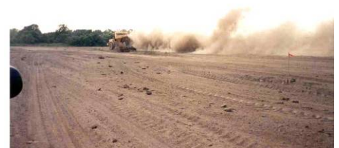
Dust can be a hazard when it blocks visibility
