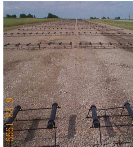
Dowel in baskets placed on the grade at joint locations prior to paving
