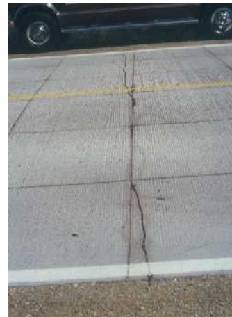
Typical late sawing crack
