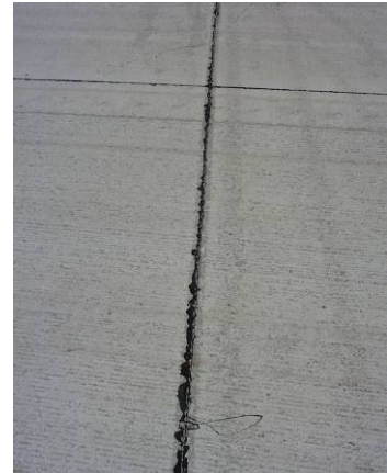
Raveled joint due to sawing too early
