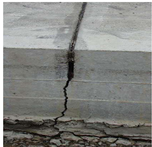
Joint sawed at the top of the pavement and cracked below
