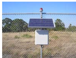
Airfield obstructions, such as fences, can be economically marked at night with mountable solar LEDs.
