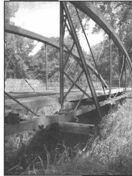
Close up view of side supports on the Coon Hunters' Bridge. Photograph by Evan Vulich 2003.
