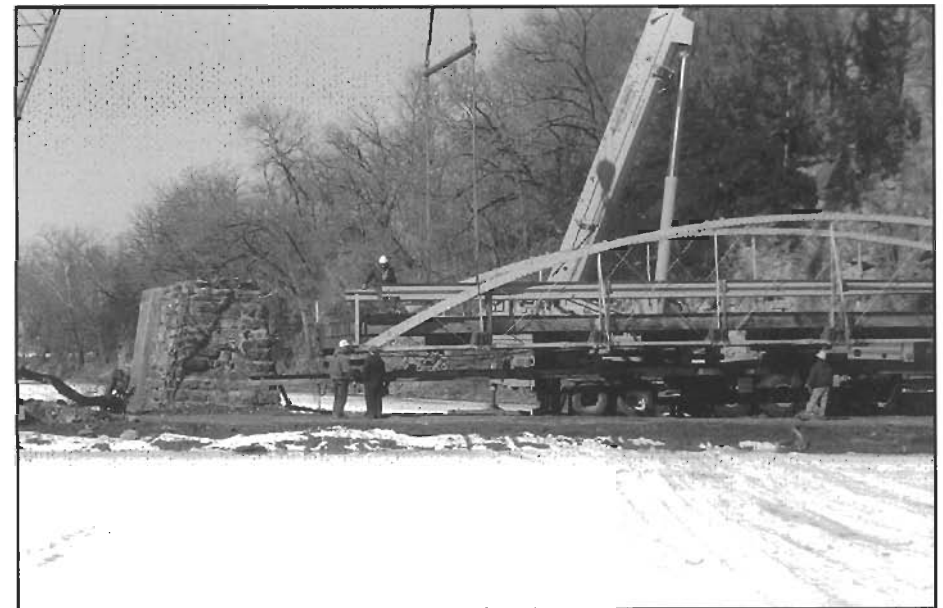
Removal of the 81 foot middle span of the Hale Bridge by Peterson Contractors, Inc. and Voss Moving Company, February 2003.
