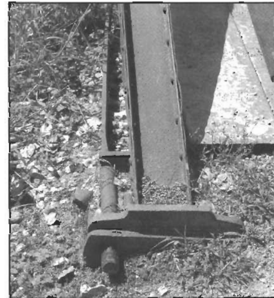
Close up view of the steel plates that anchor the Coon Hunters' Bridge to the ground. Photograph by Evan Vulich 2003.
