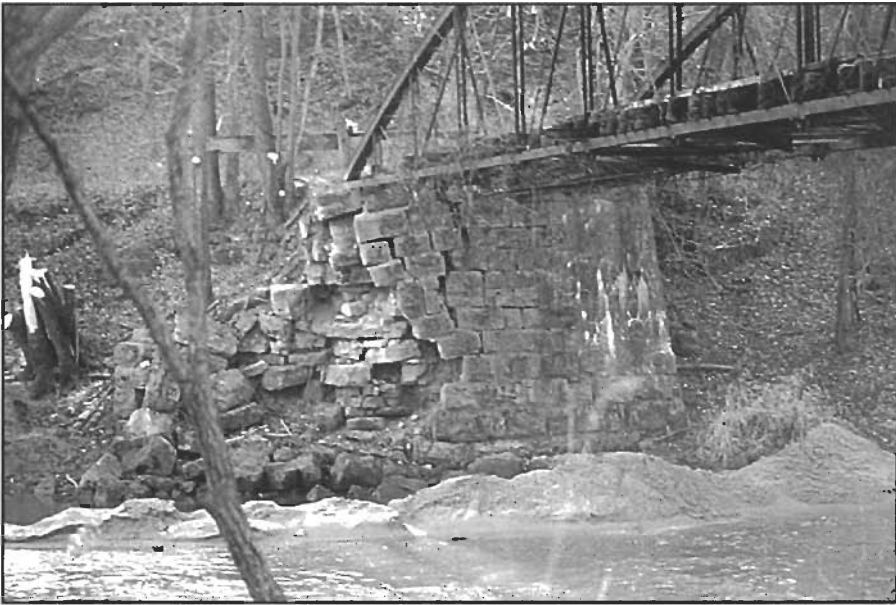
Close up of Corbett's Mill Bridge showing damage to the stone pier on the western end of the bridge prior to renovation. Photograph by the author 2001.
