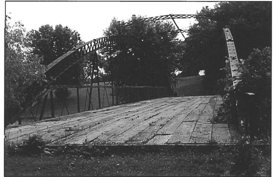
Approach to the Fremont Mill Bridge. Photograph by the author 2002. (FHWA#: none)
