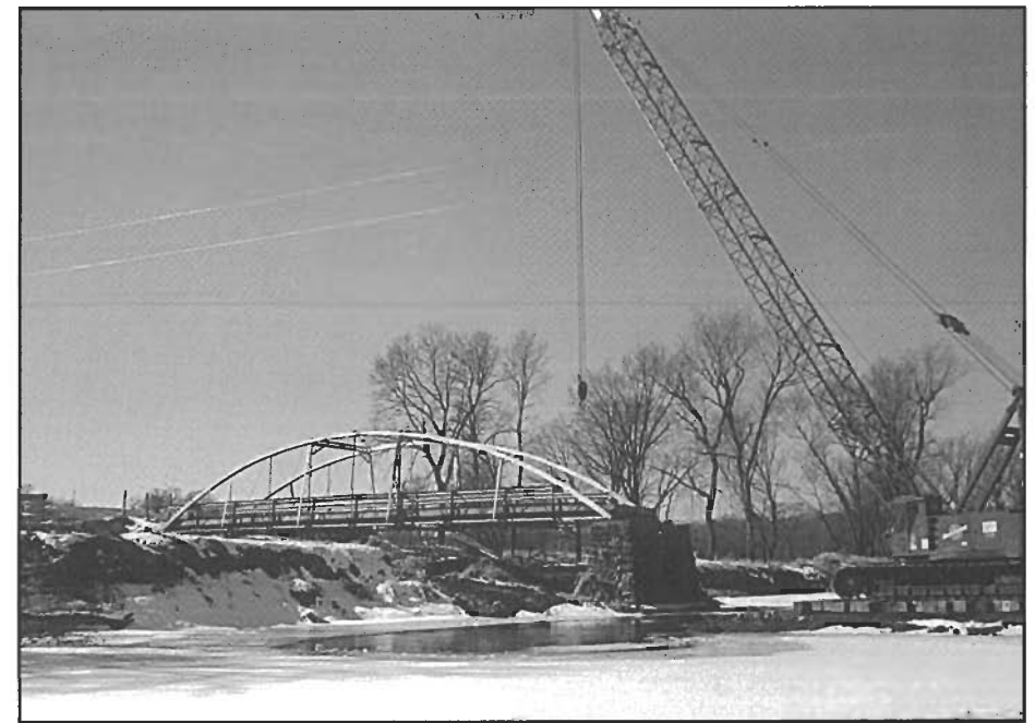
Removal of the 100 foot southern span of the Hale Bridge by Peterson Contractors, Inc. and Voss Moving Company, February 2003.
