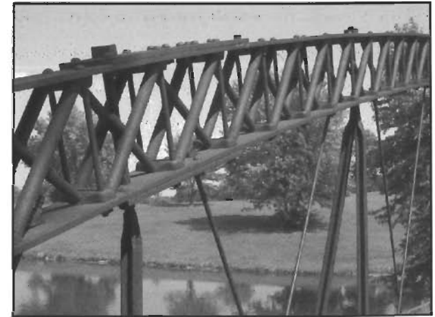
Photograph of the standard double-plated lattice design on the Fremont Mill Bridge, Jones County. Photograph by Evan Vulich 2003.
