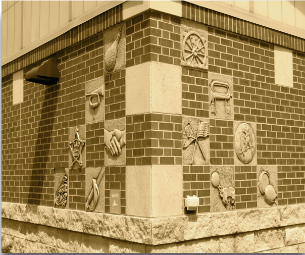
Exterior cladding on the restroom building at the southbound rest area in Franklin County on Interstate 35.
